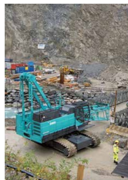
Once across the river, the CKE900G-2 was used primarily to lift 25m-long reinforcement cages for the project's piling works
