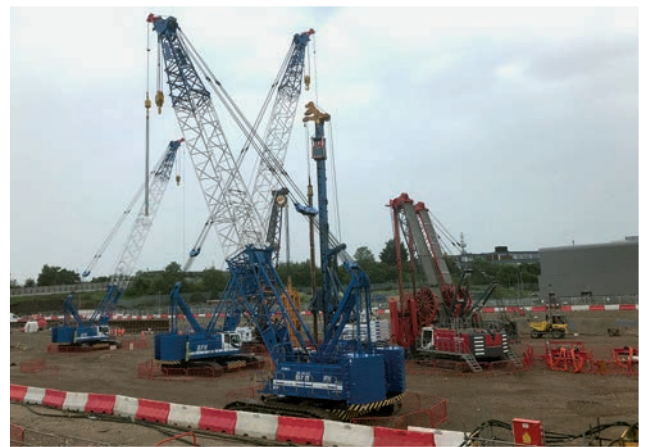
The SB3 JV is using four Kobelco CKE1350G-2 crawler cranes during construction of the £1 billion Old Oak Common main station box's diaphragm walls and associated structures.
