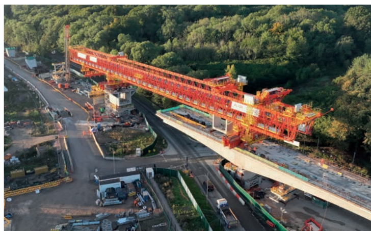
Construction of HS2's 3.4km-long Colne Valley Viaduct, between Hillingdon and the M25, is using a 700 tonne, 160m-long 'launching girder', and will be the longest railway bridge in the UK when complete in 2025.
