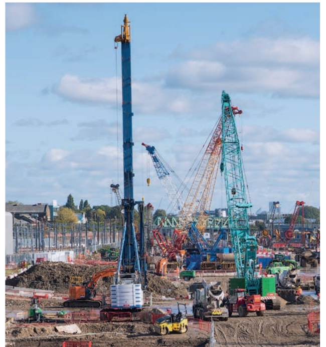
BPH Equipment's CKE900G-3 crawler cranes are using Kobelco's KCross remote operation management system to monitor working conditions, location, maintenance history and fuel usage during operation at Old Oak Common station build.
