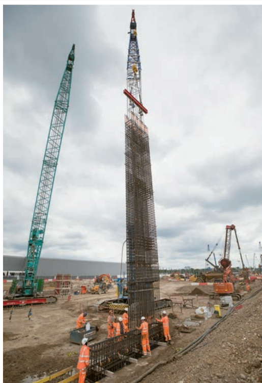
One of SB3's four Kobelco CKE1350G-2 lifting rebar during construction of HS2's Old Oak Common station box's 1.8km-long, 25m-high diaphragm walls, and associated structures.
